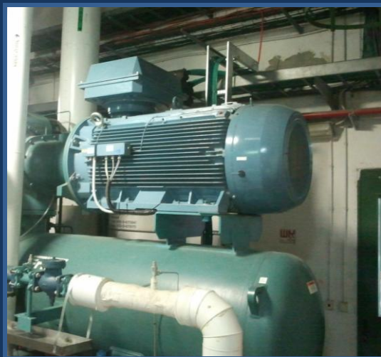
Figure 1a: 700 HP, 400V/50 Hz Cooling Compressor - Carlsberg
