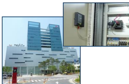
EG4K Installation at LG IDC, Seoul Korea
